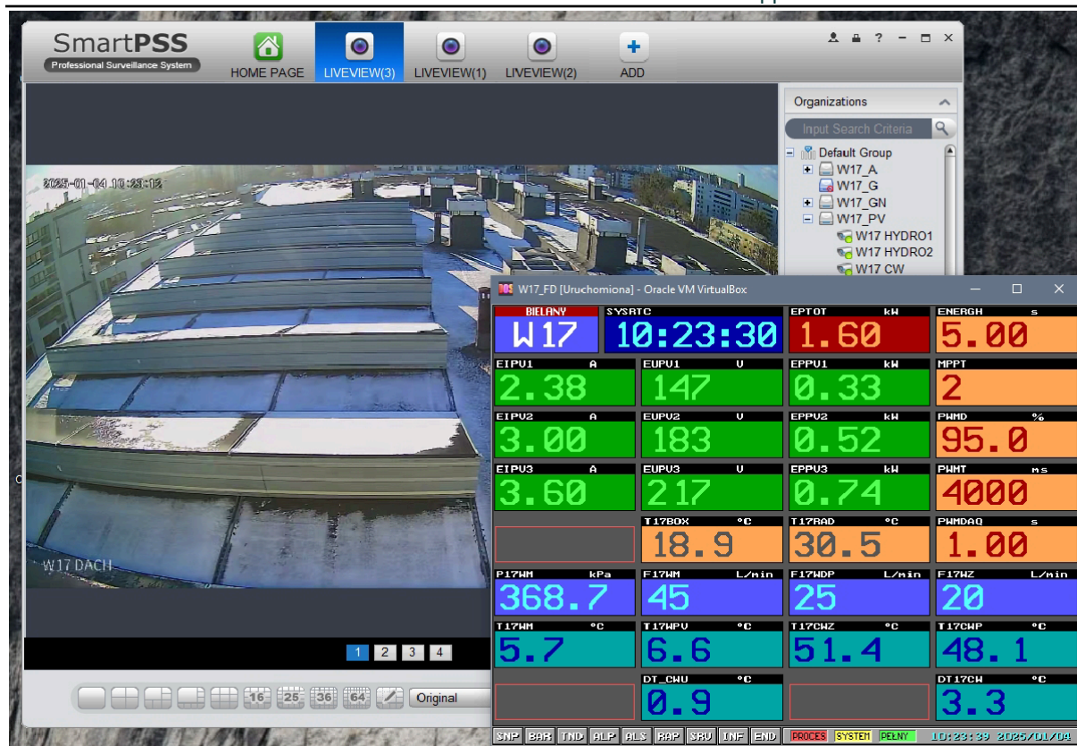
Figure 2. SCADA system monitoring photovoltaics on the roof
